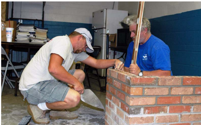
Here, Chipola masonry instructor Melvin Dawson (right) assists apprentice student Robert Pugh of Panama City as he performs brick-laying exercise in the masonry lab.
